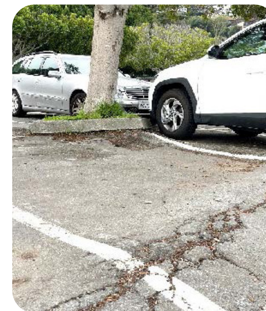
Heaving and cracks caused by fig tree roots
